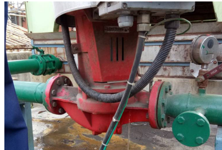
FIGURE 2: WATER LEAKAGE FROM RUSTED CASING, WITHOUT E-COATING
